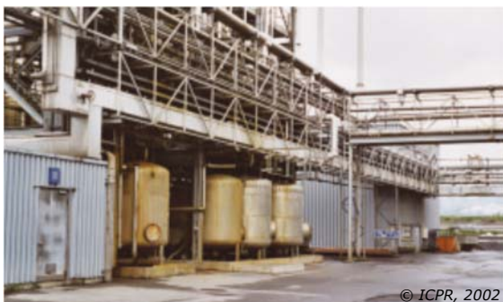
Storage of fixed tanks
